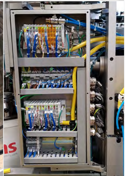
Cooling of control cabinets
